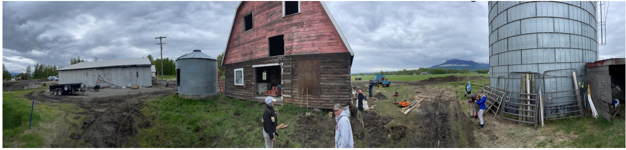
Attachment 1: Panoramic photo of the barn during initial efforts to restore it. The faded paint and lack of a proper foundation are clearly visible.
