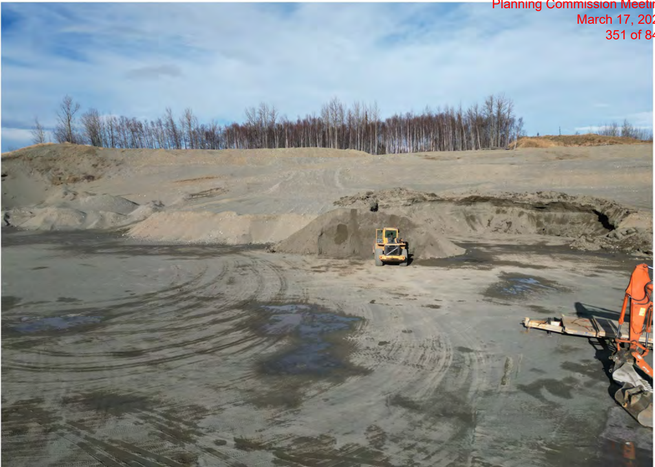
View to north, pit floor in foreground with front loader and working face of Phase 1 to right.
