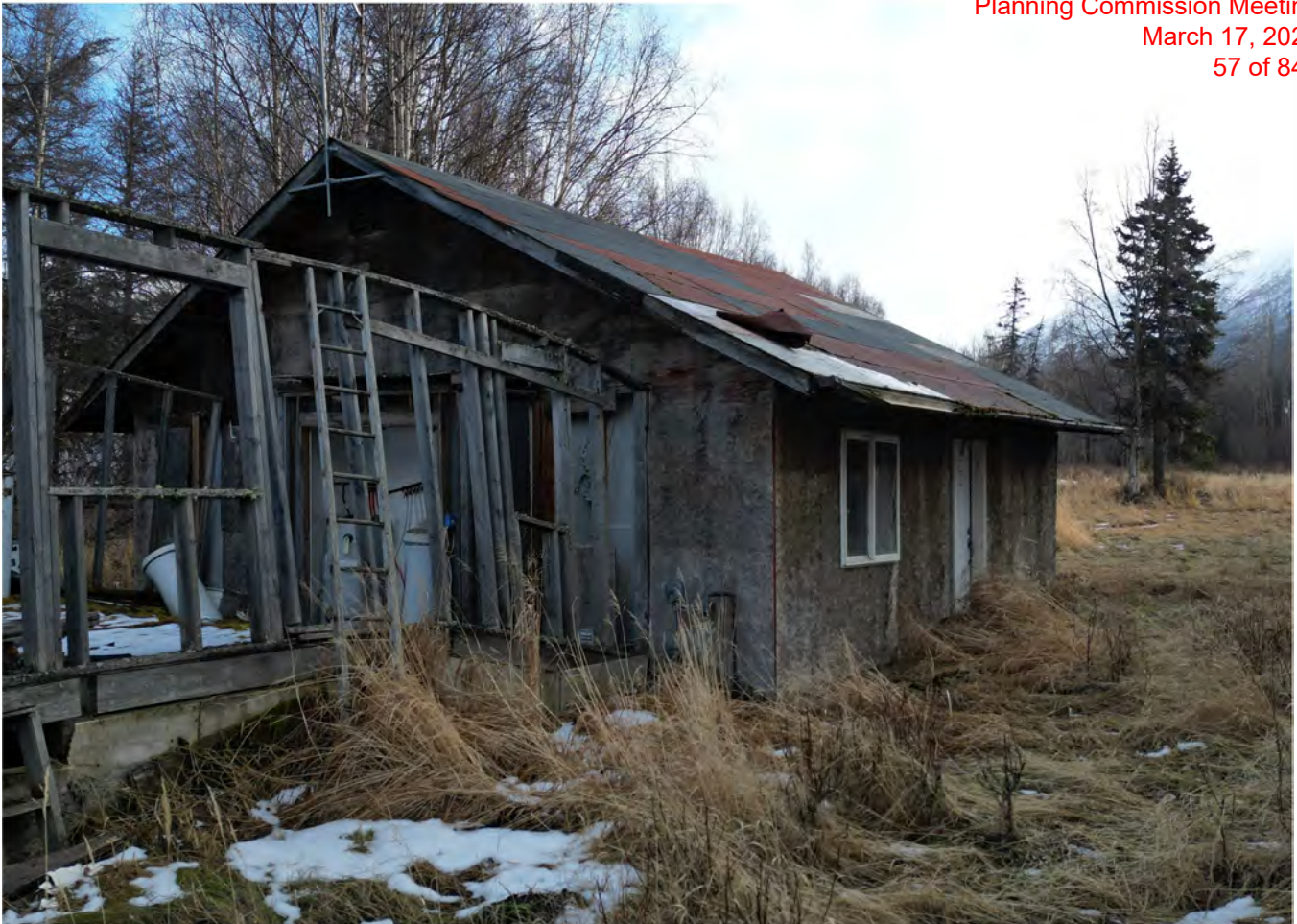
Derelict residential structure on subject property. Ground view to southeast.
