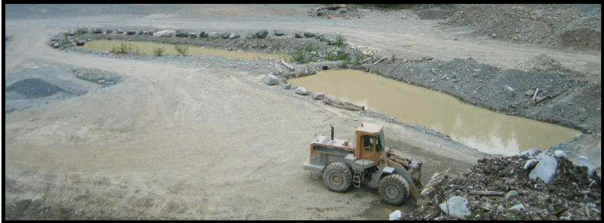
Figure 7-15: Settling Pond Example (Photo: City and Borough of Sitka)
