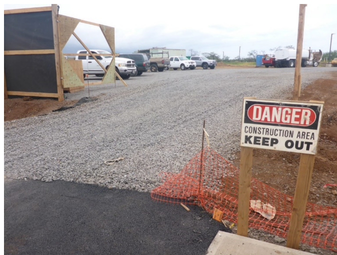
A construction entrance stabilized with gravel over filter cloth reduces the amount of sediment transported off site.
