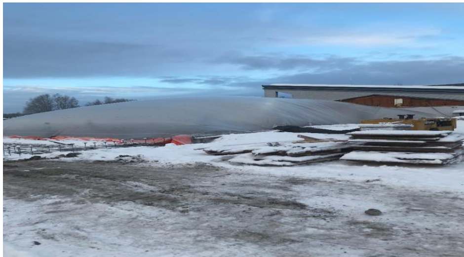
Above Photo: Old Willow Library Demolished and Site Covered for New Construction
