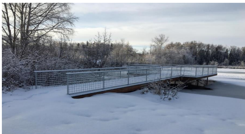
Above Photo: New Big Lake Fish Viewing Platform with handrail structure and mesh pedestrian panels
