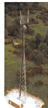
Right: Communication tower
