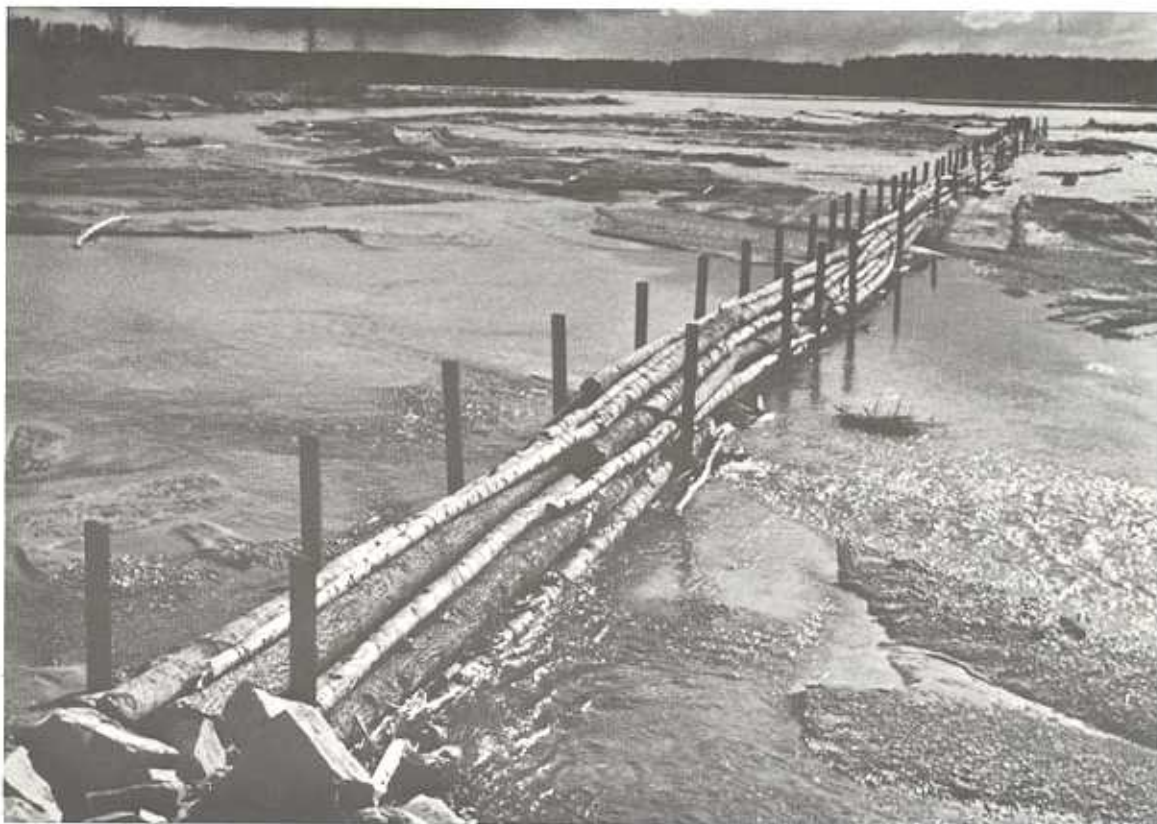
VIEW OF FASCINE FROM UPSTREAM END AS IT APPEARED IN MAY, 1951 FIGURE 4
