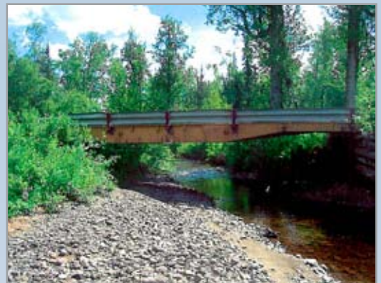
This "bridge" is actually the flatbed of a railcar with the wheels knocked off.
