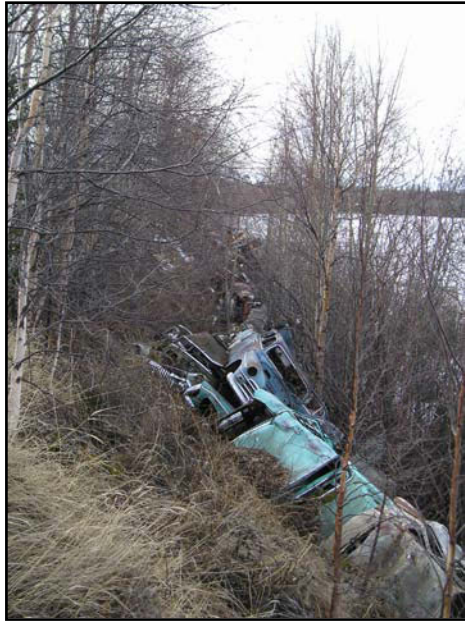
Junk cars have been used unsuccessfully and illegally by private property owners in an attempt to slow erosion along lower reaches of the river.
