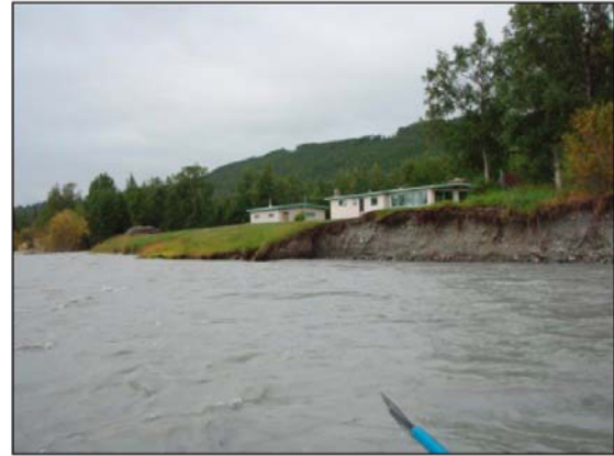
The residents of this Sutton home have taken immaculate care of the property since 1959 as the Matanuska River continues to advance.
