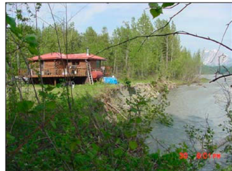
2006 view of one of three homes in Sutton that was included in the Emergency Watershed Protection Program buyout administered by the USDA Natural Resources Conservation Service with MSB Assistance.
